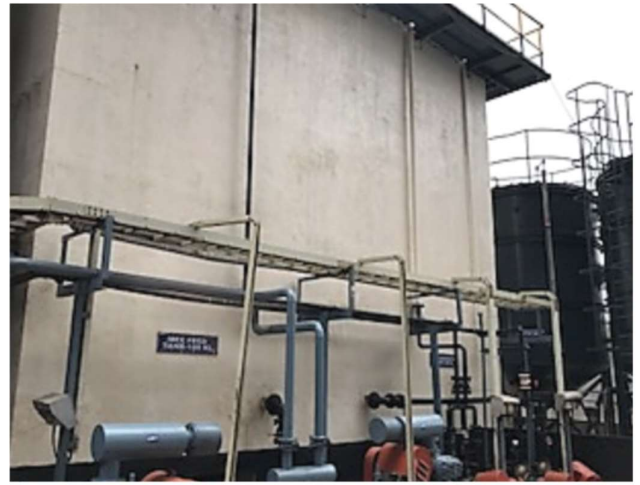
Above ground level effluent tank
