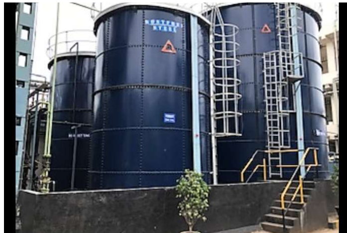
Effluent storage tank (Above the ground) & Secondary containment
