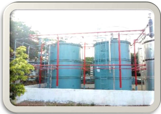
Chemicals storage tanks (Above the ground) & Secondary containment
