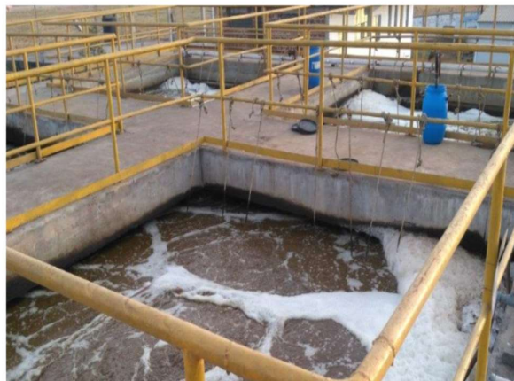
Biological treatment plant
