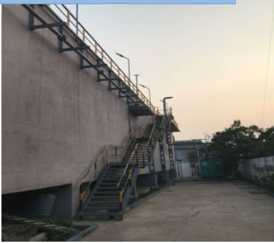
Above ground level effluent tank
