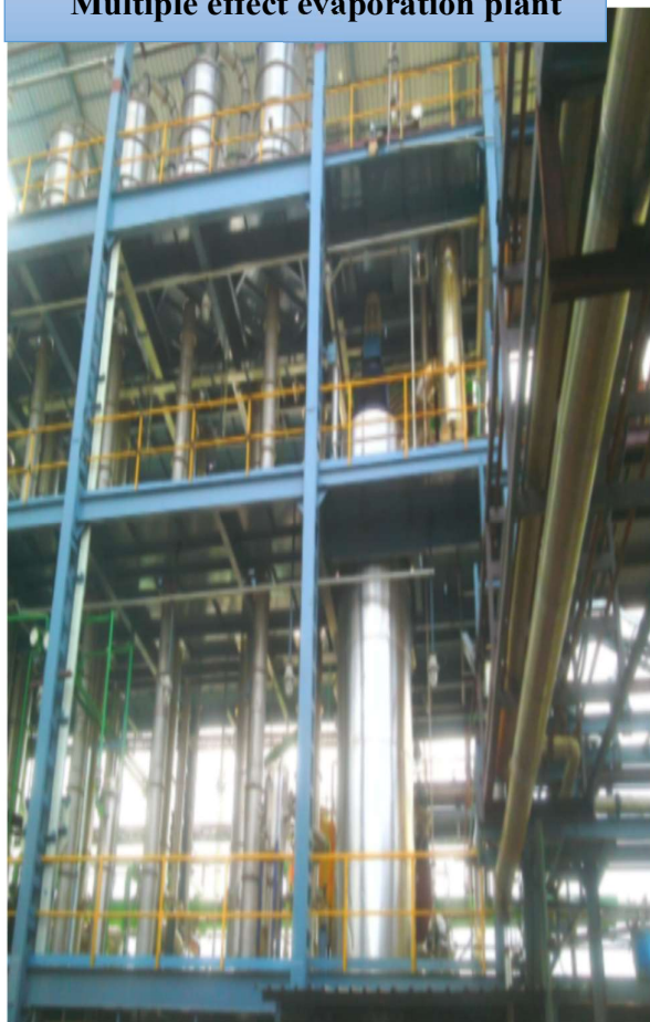
Multiple effect evaporation plant
