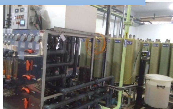
Reverse Osmosis (RO) system
